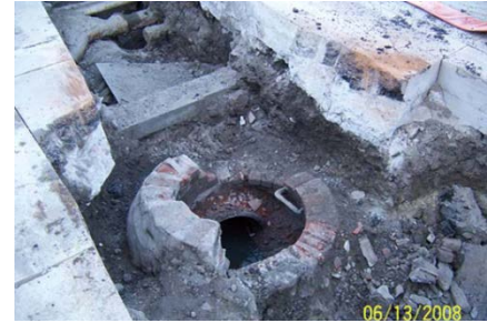
Emergency repair of old collapsed sanitary sewer manhole in North Main Street, June 2008.
