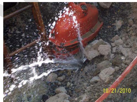
Water main break on South Main Street, October 2010.
